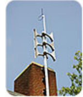
Cooper Notification's WAVES High Power Speaker Array is installed at Virginia's James Madison University.
